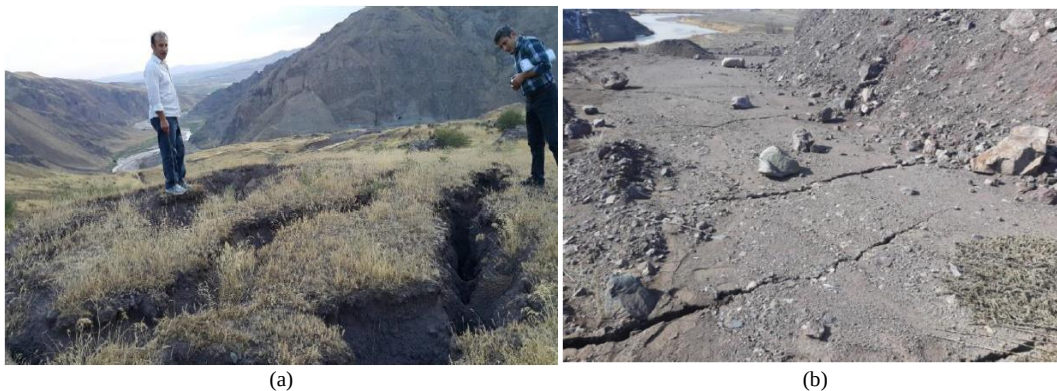
Figure 2 - a) Cracks created near the slippery toe caused by local instabilities in the toe. b) Tensile cracks created in the coated materials forming the downstream slopes of the bridge
